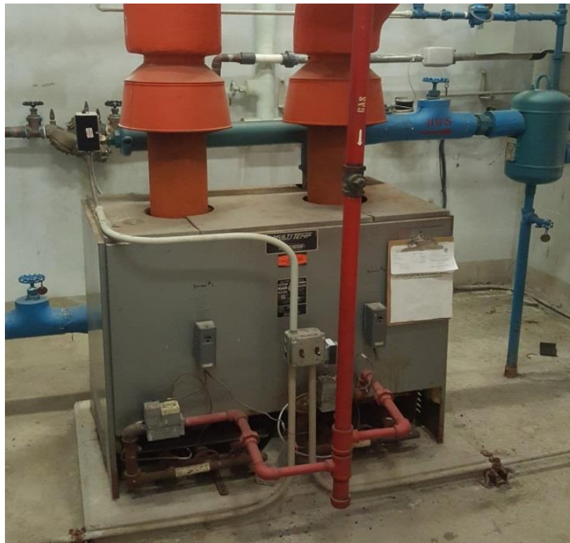
Control Building Boiler
