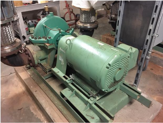
Typical BHS Pumpset
