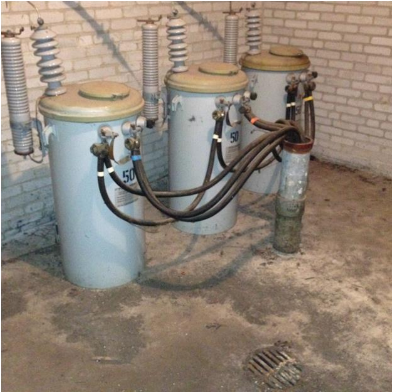
Typical Underground Transformer Vault
