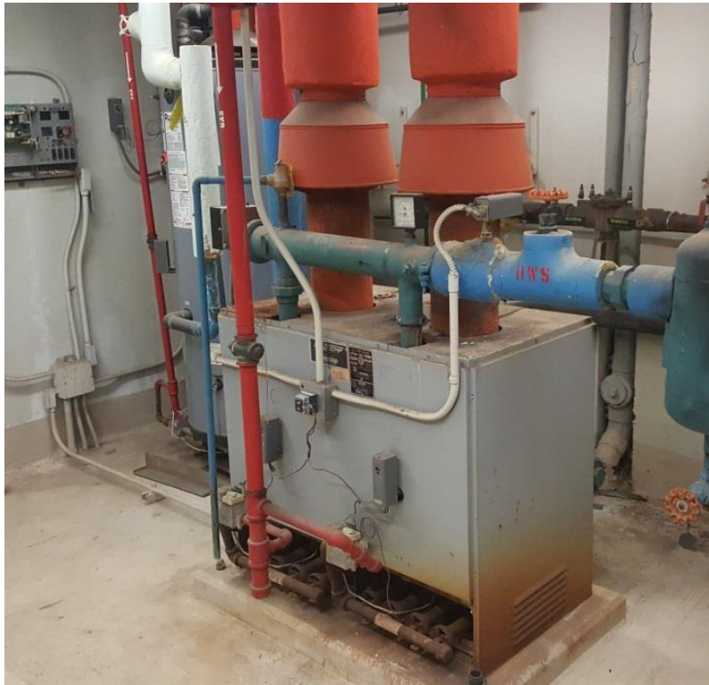
Mechanics Building Boiler
