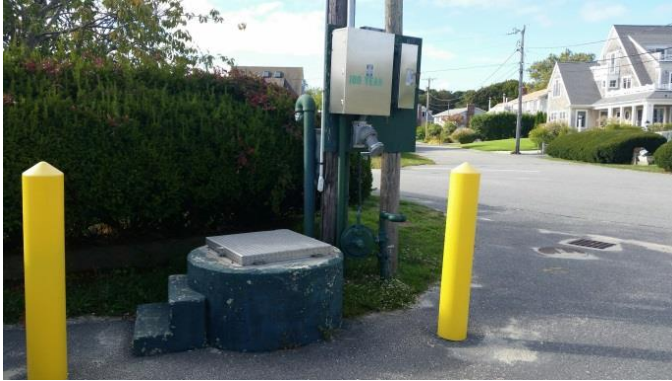
Bayshore Road Pump Station
