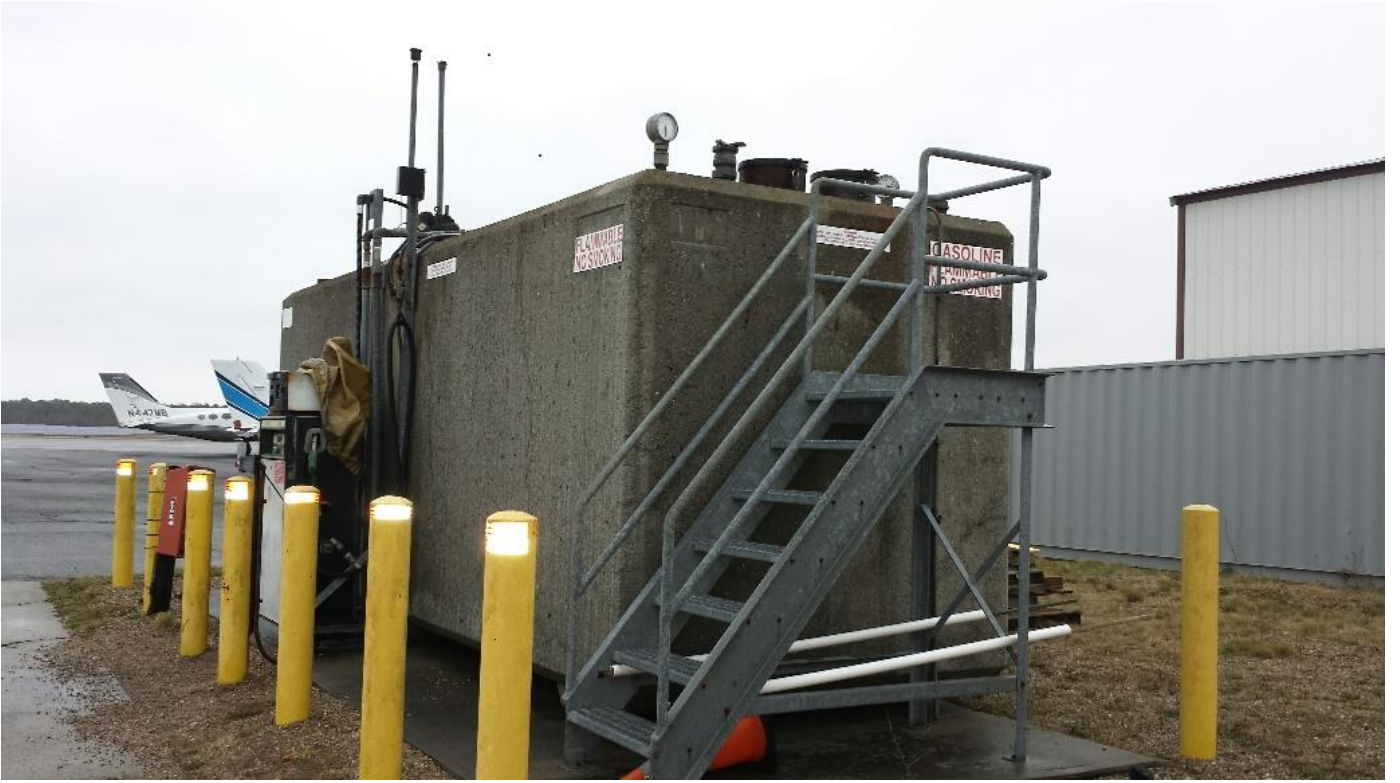
Mo-Gas and Diesel Fuel Con-Vault, Gas Boy & Alarm
