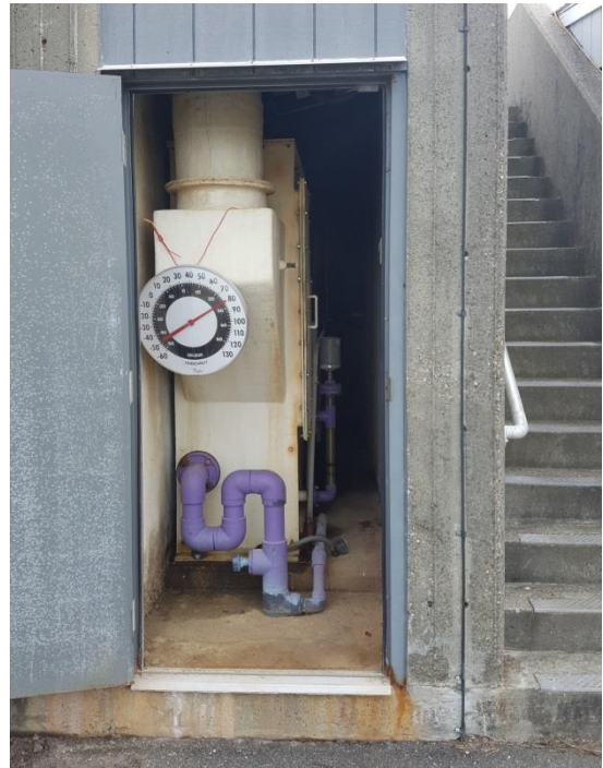
Odor Control System Access
