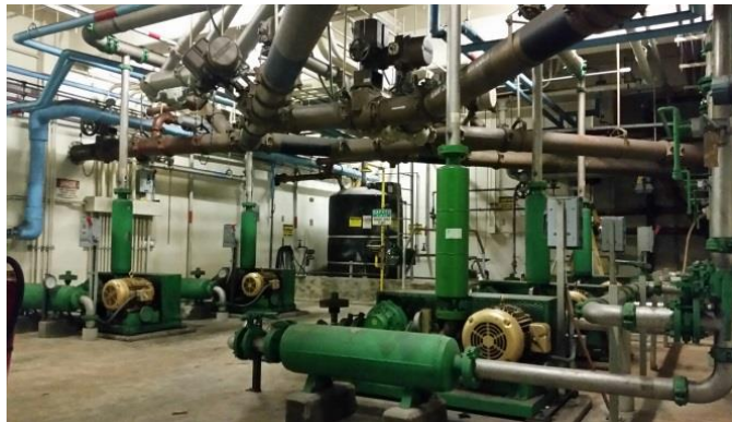
Septage Blower Room
