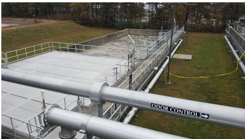
North Aeration Tank
