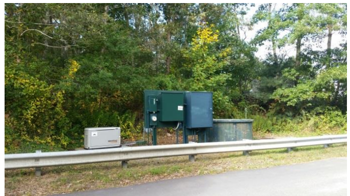
Oak Neck Road Pump Station
