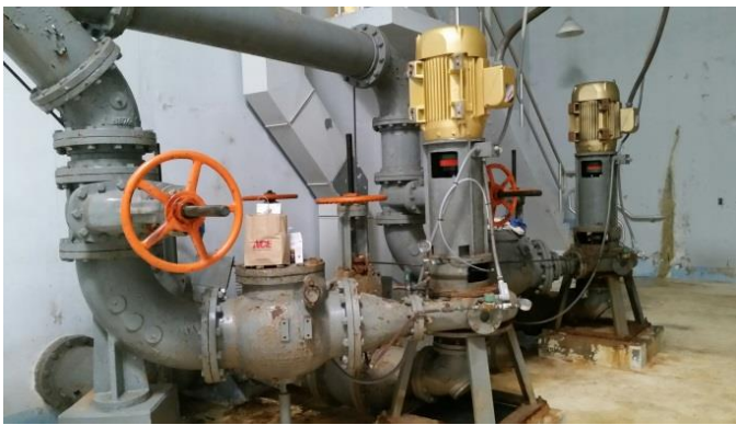
Freezer Road Pump Room
