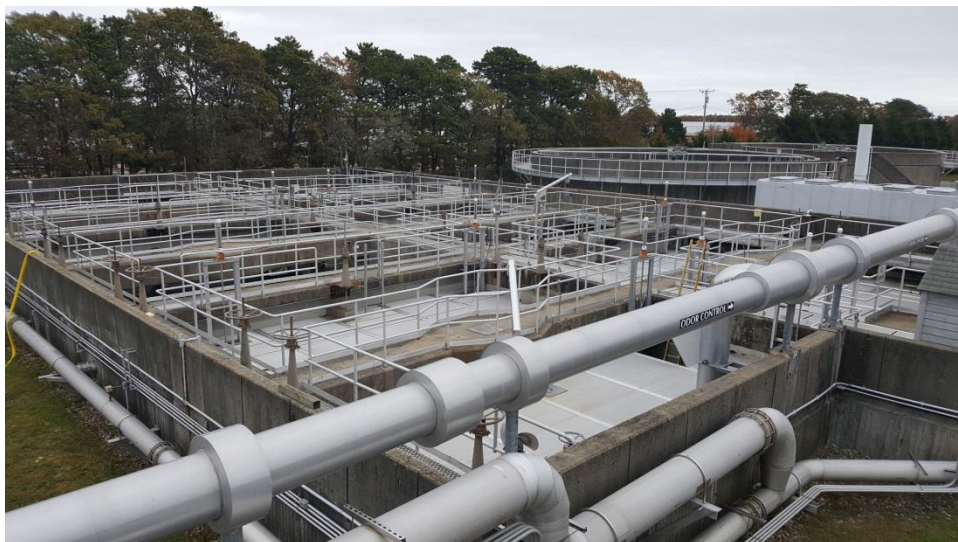
Middle and South Aeration Tanks
