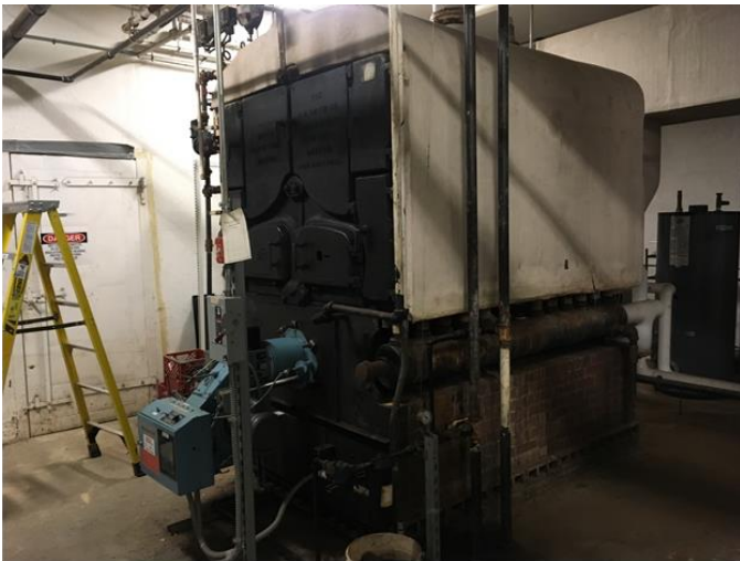
Barnstable West Barnstable Elementary School Boiler
