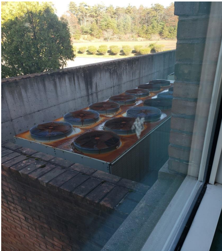
Barnstable United Elementary School Chillers
