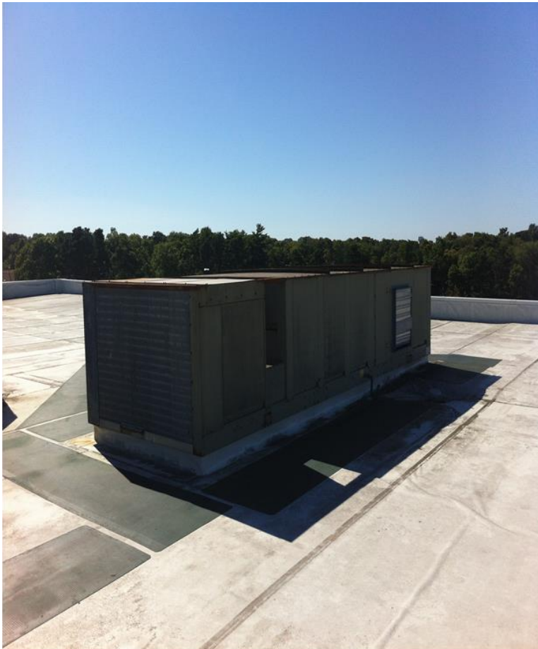
Roof Top Units (RTU)
