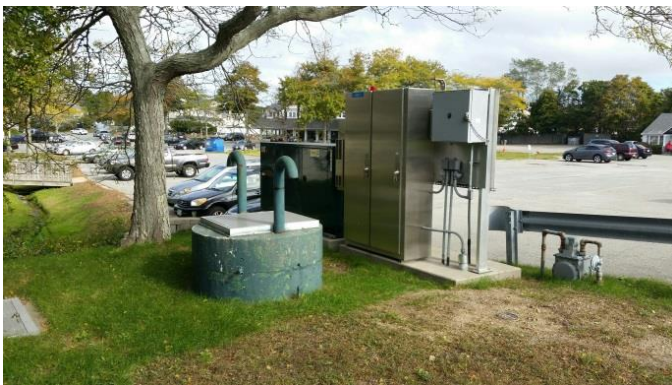
720 Main Street Pump Station
