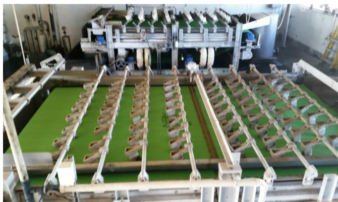
Sludge Thickening Belt
