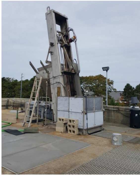
Mechanical Bar Screen
