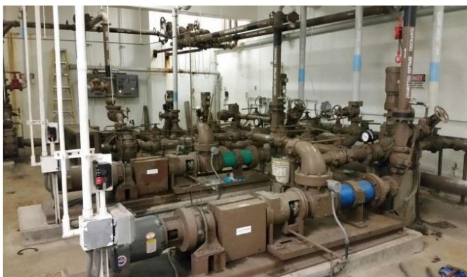
Sludge Pump Room
