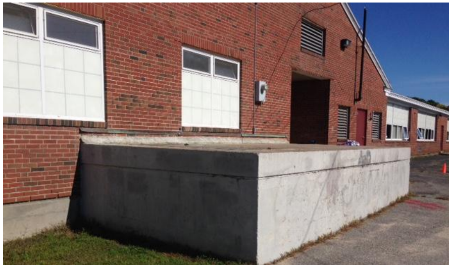
HYW Transformer Vault
