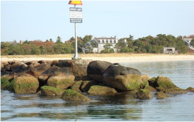
Breakwater Damaged by Storms
