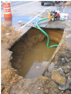
Barnstable Road Failing Water Main
