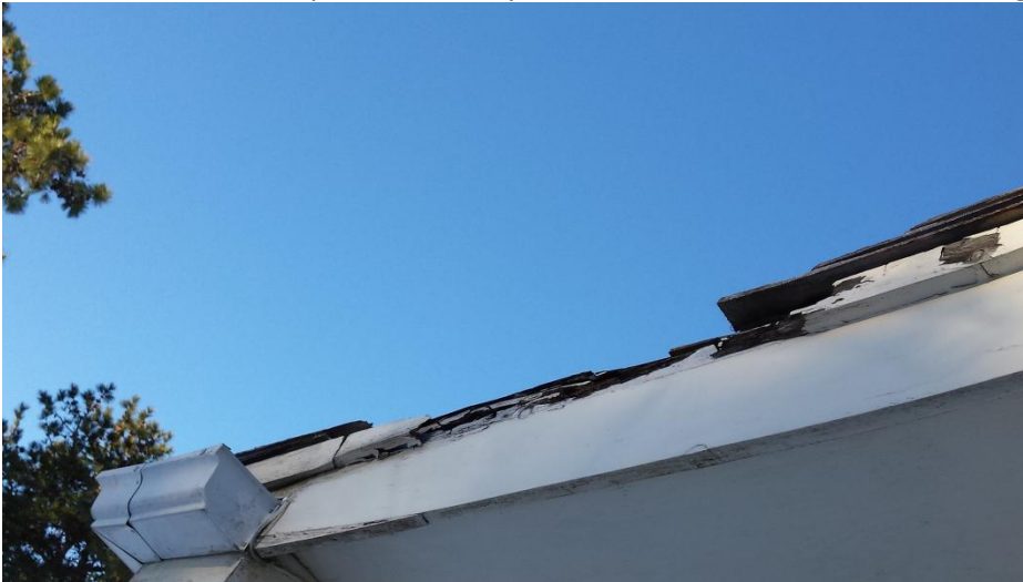
Clubhouse Roof Trim
