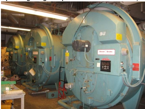
High School and Middle School Boilers
