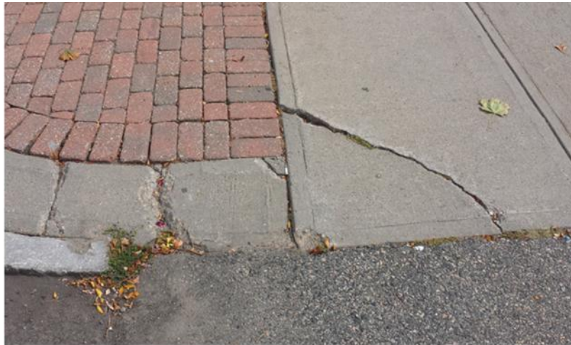
Main Street Hyannis Sidewalk Hazardous Conditions
