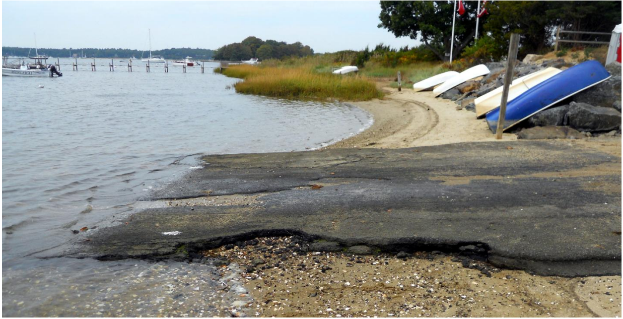
Deteriorated Boat Ramp
