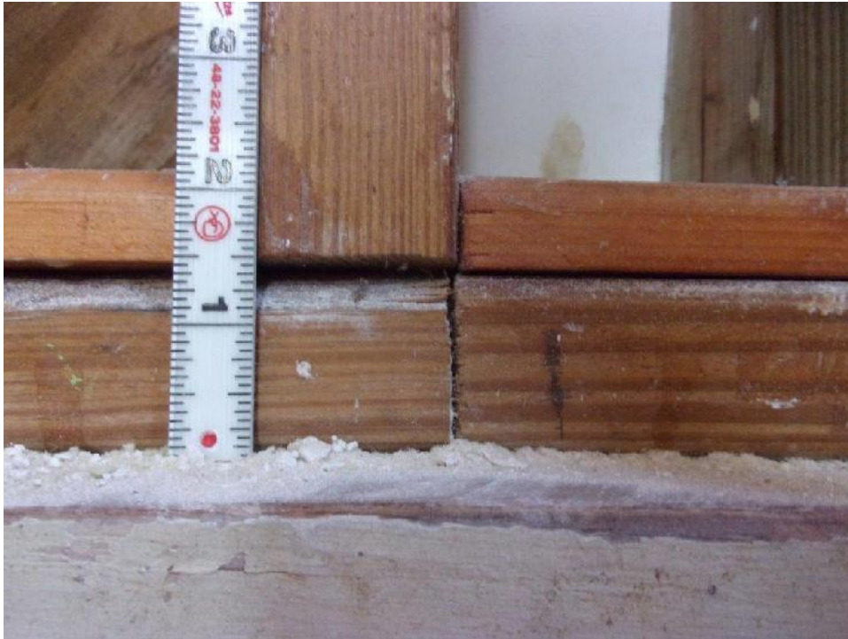
Typical discontinuous second floor exterior wall sole plate joint with no mechanical attachment observed
