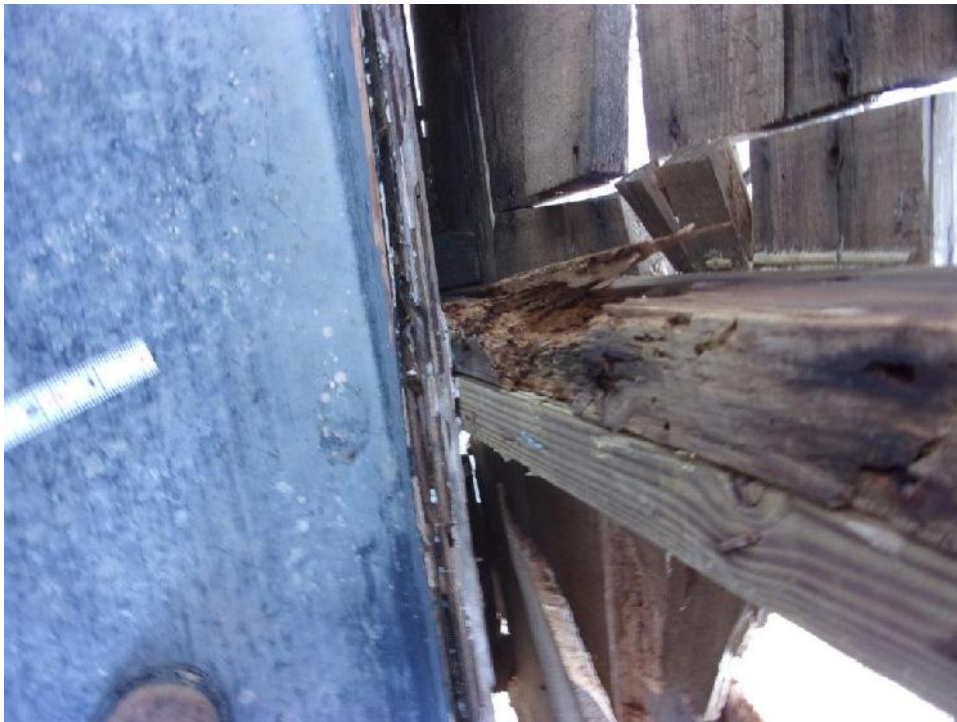
Typical rotted/deteriorated second floor wrap-around balcony board sheathing and exterior railing post; constructed with dimensional lumber
