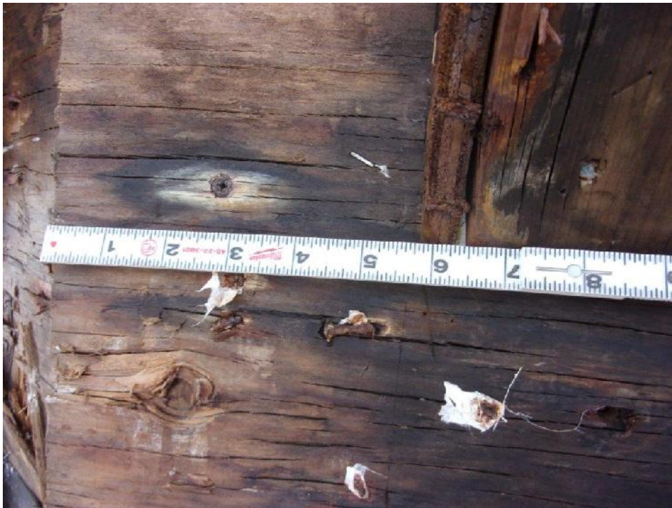
Typical second floor wrap-around balcony with separation of sheathing from diagonal support; constructed with dimensional lumber
