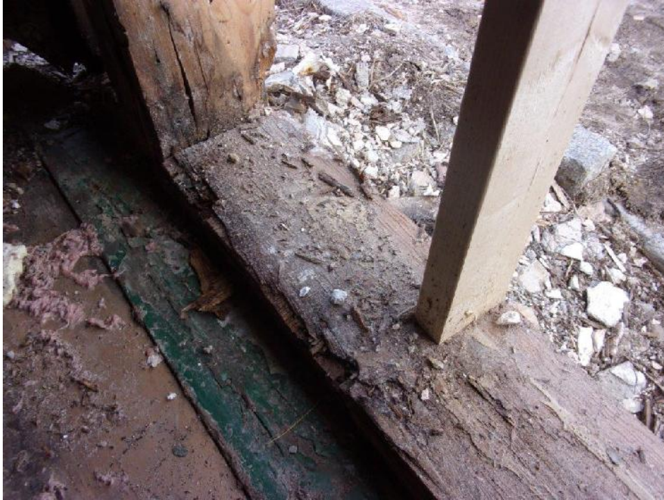
Typical deteriorated first floor sole plate at exterior wall (in contact with foundation); no mechanical fasteners connecting sole plate to foundation
