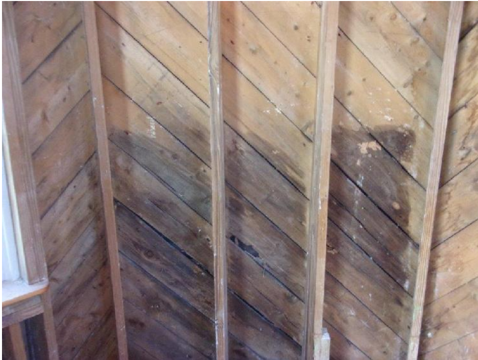
Typical third floor board sheathing with visible water staining and deterioration; constructed with dimensional lumber
