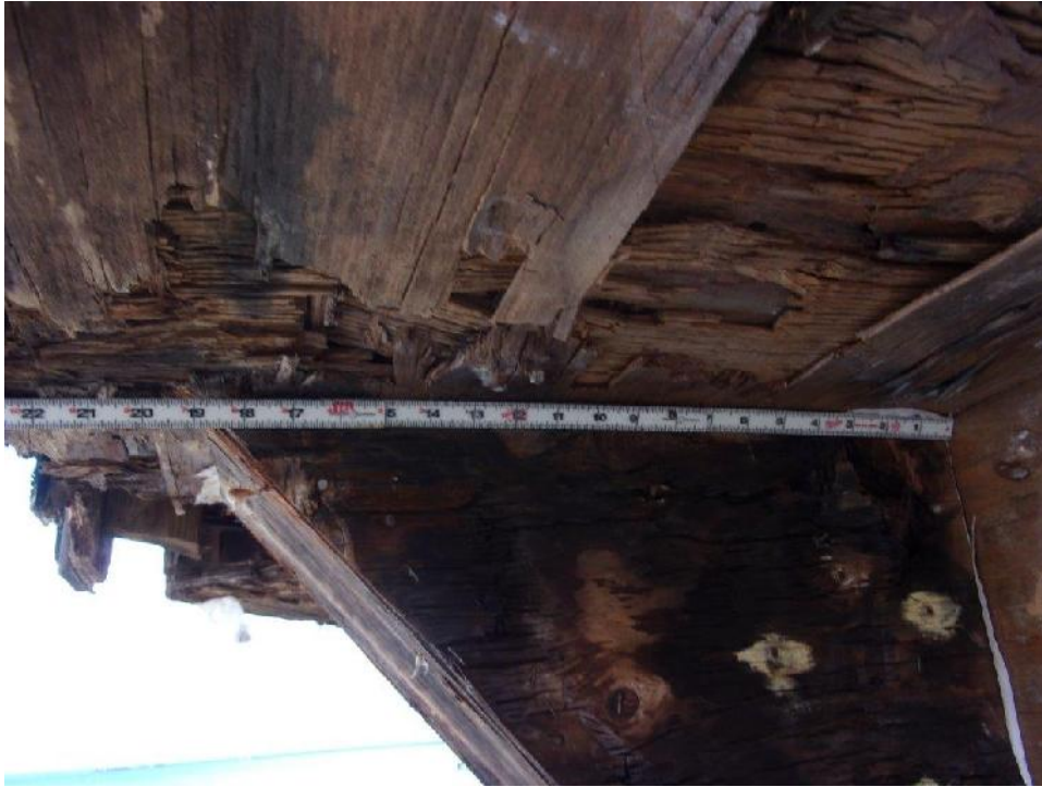
Typical underside of second floor wrap-around balcony with failed sheathing (layers separating); constructed with dimensional lumber
