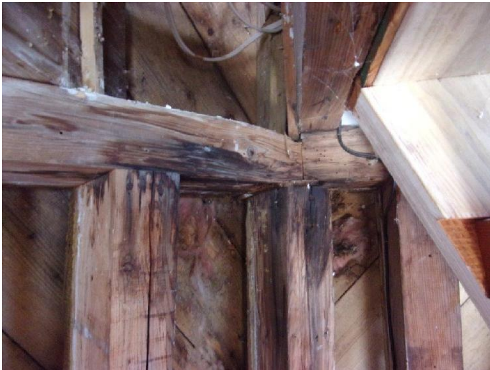
Second floor exterior wall framing with visible water staining, rot & crushing of top plate
