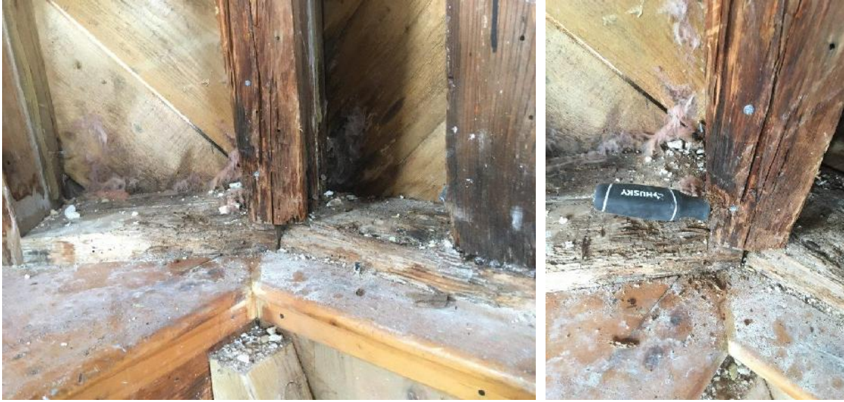
Typical second floor exterior wall stud rot/deterioration at sole plate of second floor exterior wall
