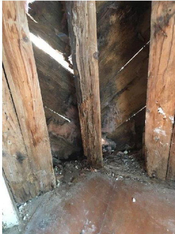
Typical second floor exterior wall stud and wall board with evidence of staining and deterioration
