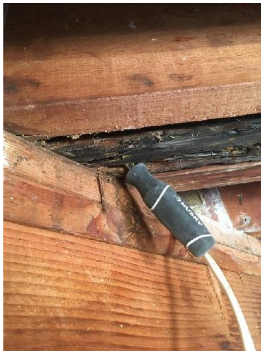
Typical deteriorated second floor beam end supported on supplemental interior framing
