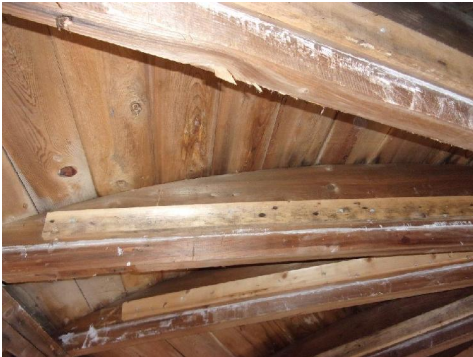
Typical dome roof framing curvature and board sheathing with visible signs of water staining
