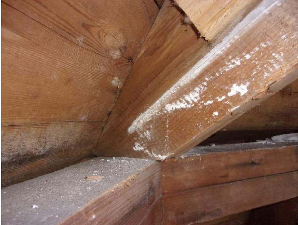
Typical dome roof framing support at double top plate at third floor exterior wall; no mechanical fasteners observed
