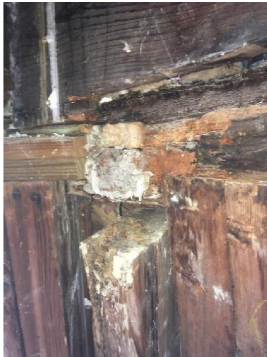
Typical second floor wall stud fully separated top plate; no longer providing support to gravity load resisting system
