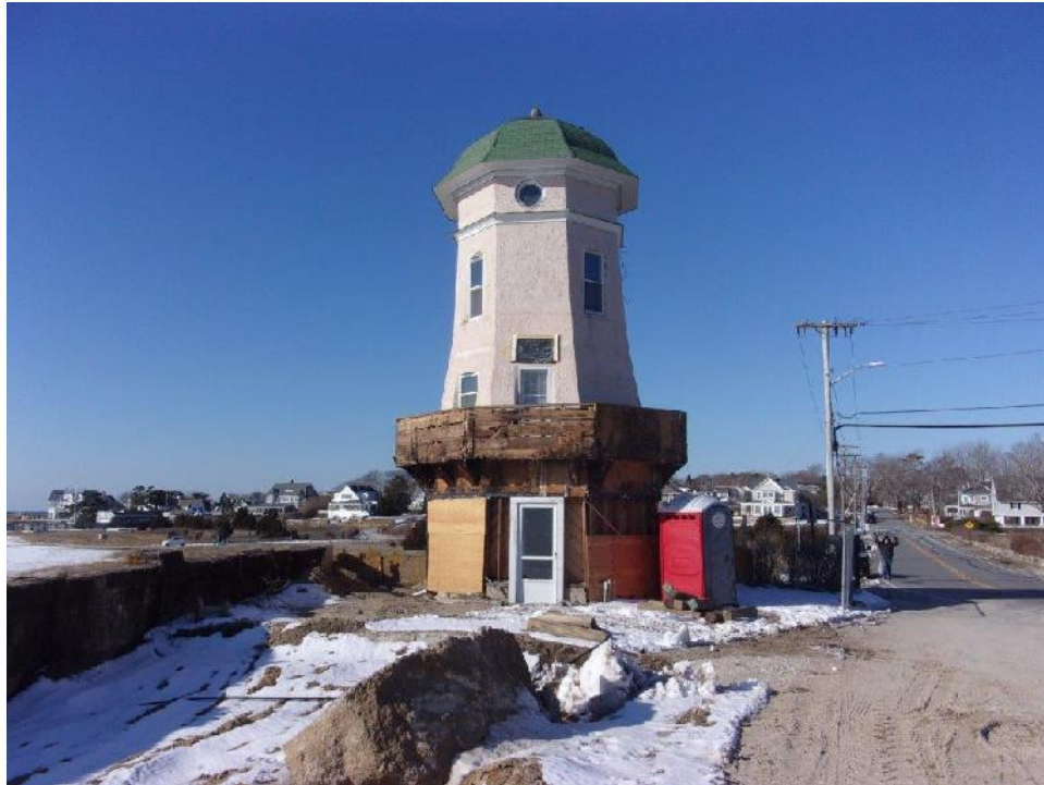
Overall structure elevation looking west with noticeable tilt to the southwest
