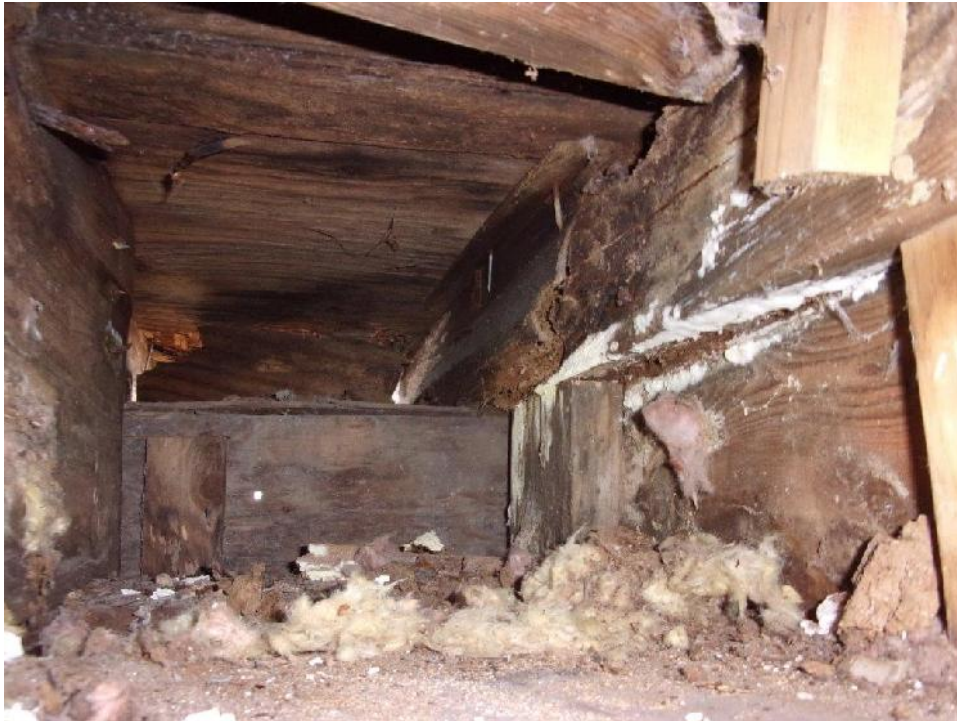
Typical deteriorated cantilever support beam for wrap-around exterior balcony at first floor exterior wall top plate (underside)
