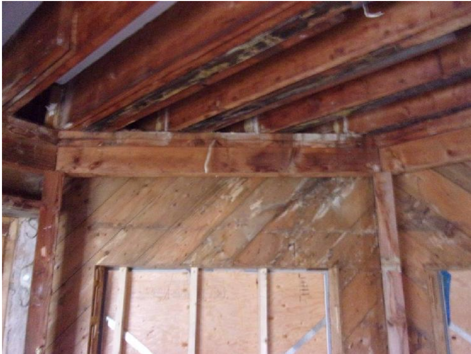
Typical second floor supplemental support framing with sporadically fastened, sistered floor beams; no mechanical fasteners connecting supplement interior framing
