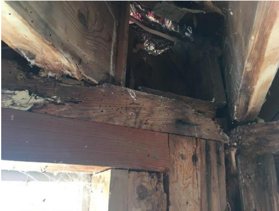
Third floor beam with evidence of insect infestation and bearing failure at second floor exterior wall top plate; deterioration/rotting visible along top plates
