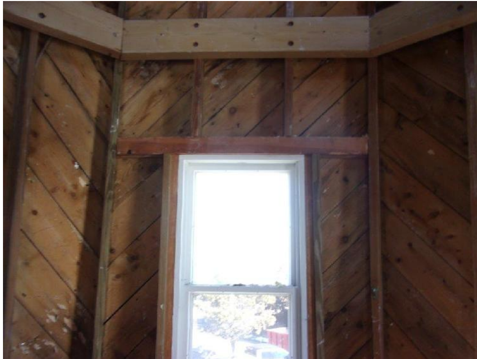
Typical third floor window header and tension/compression ring wood framing; tension/compression ring framing secured with carbon steel fasteners
