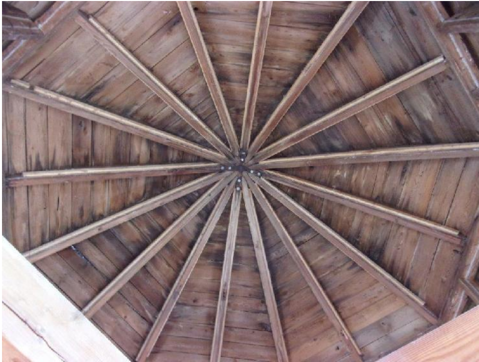
Typical existing (original) dome roof framing with visible water staining at third floor
