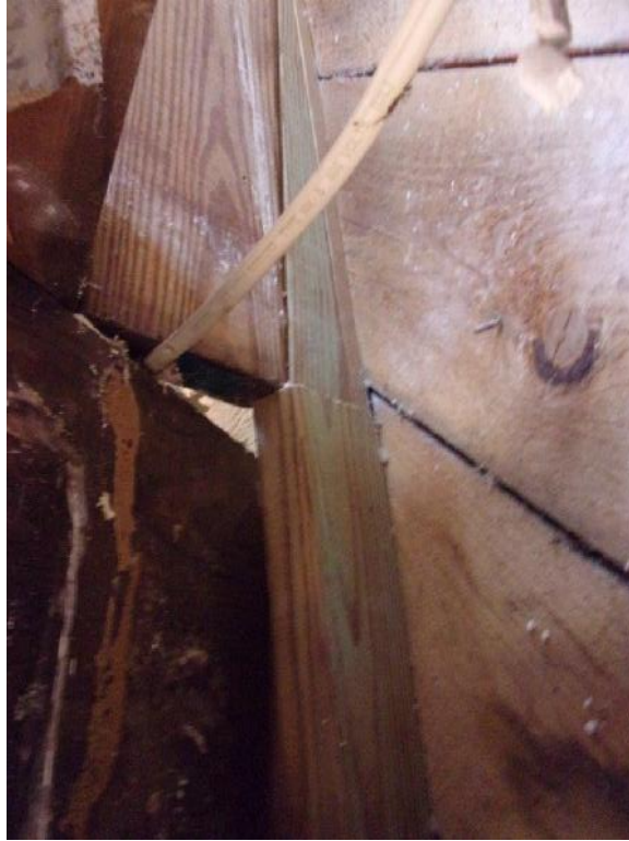
Typical third floor exterior wall stud and “wedge” not fully supported; mechanical fastening of wedges to studs not observed
