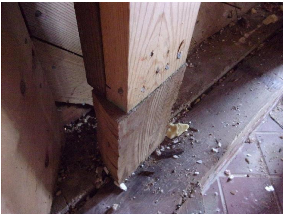
First floor supplemental framing with discontinuous column framing; no mechanical fasteners securing column base to foundation
