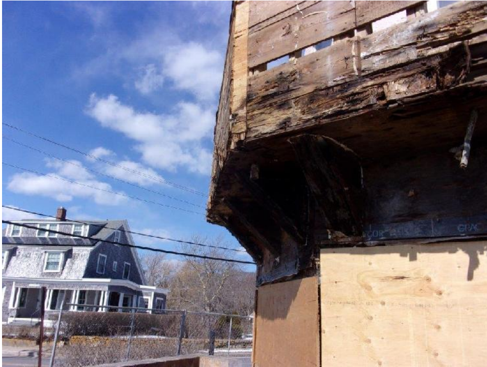
Typical second floor wrap-around balcony sheathing and supports; constructed with dimensional lumber
