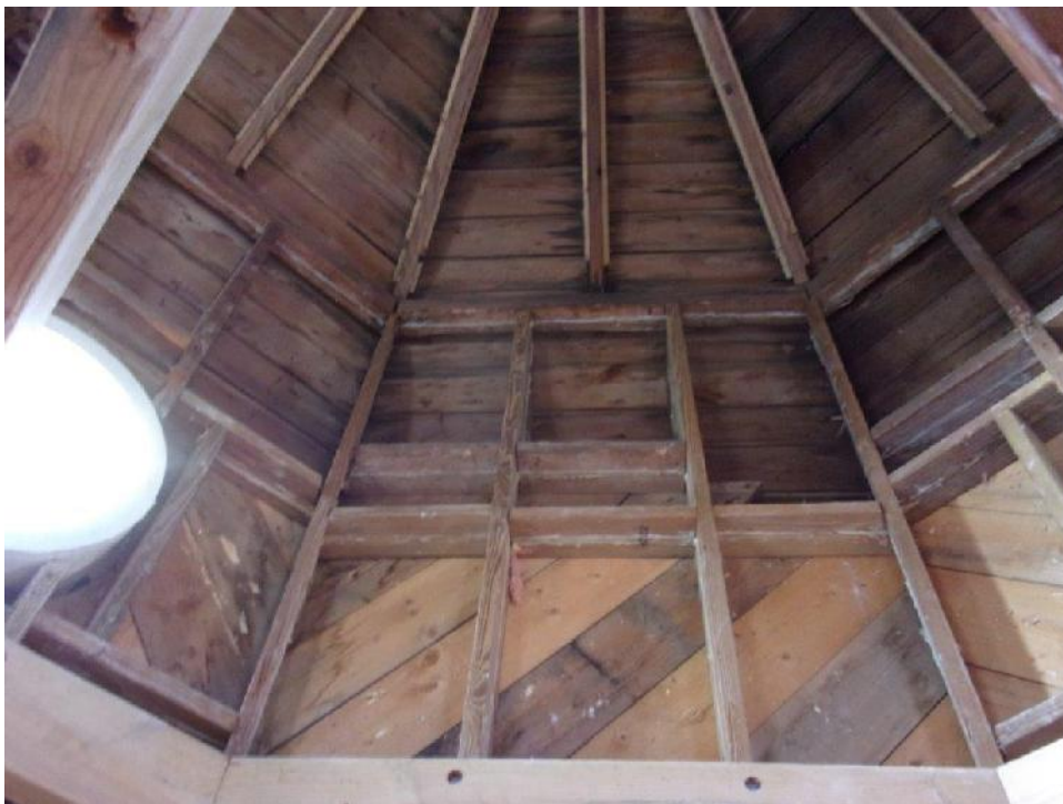
Visible discontinuous bridging at dome roof eave at third floor exterior wall framing
