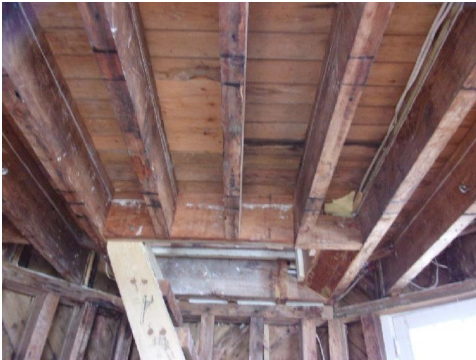
Typical third floor support framing with discontinuous header at stair opening framing at third floor
