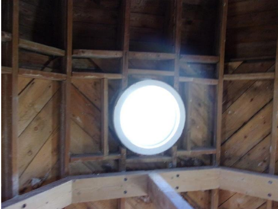
Typical third floor exterior wall framing at portal window; no jack or king studs installed (discontinuous gravity load path); constructed with dimensional lumber
