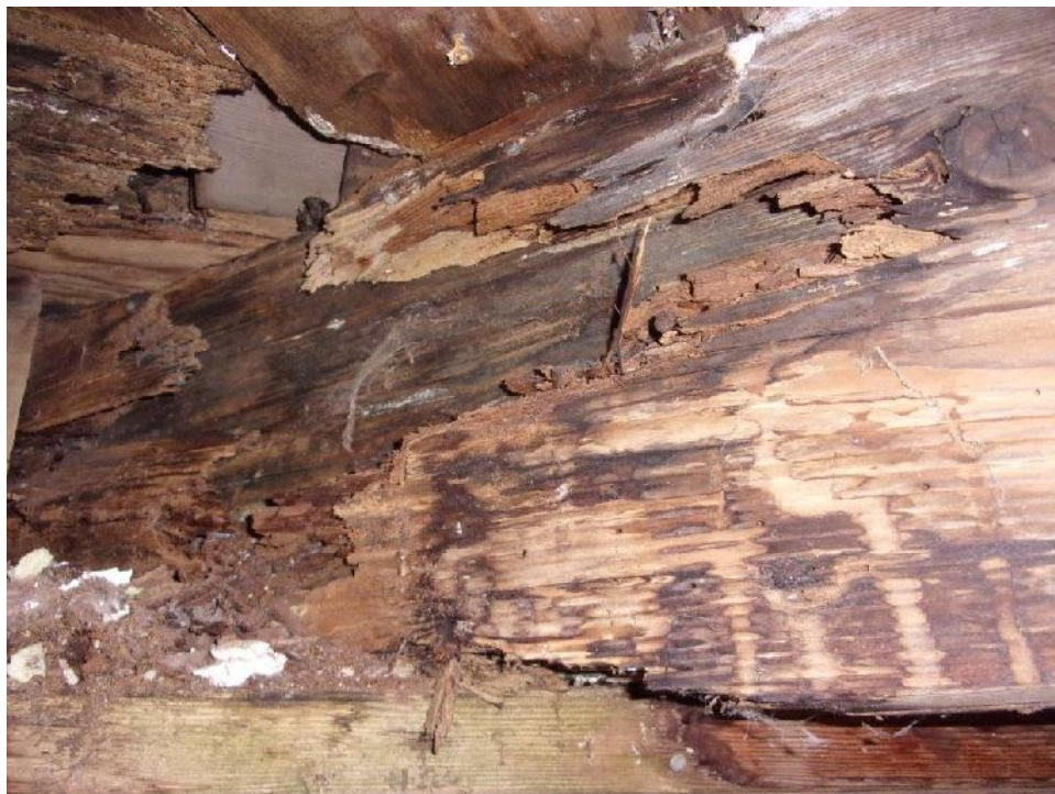
Typical deteriorated/rotted end of second floor support beam at first floor exterior wall top plate
