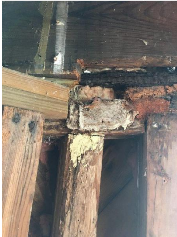
Rotted/deteriorated steel plate and wood top plate installed at second floor exterior wall
